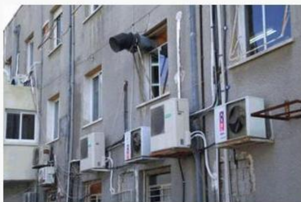
Air conditioning uses up scarce resources especially during hot weather.
